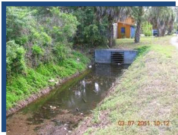
Photograph 25 South Ditch Facing East Where It Exits Park
