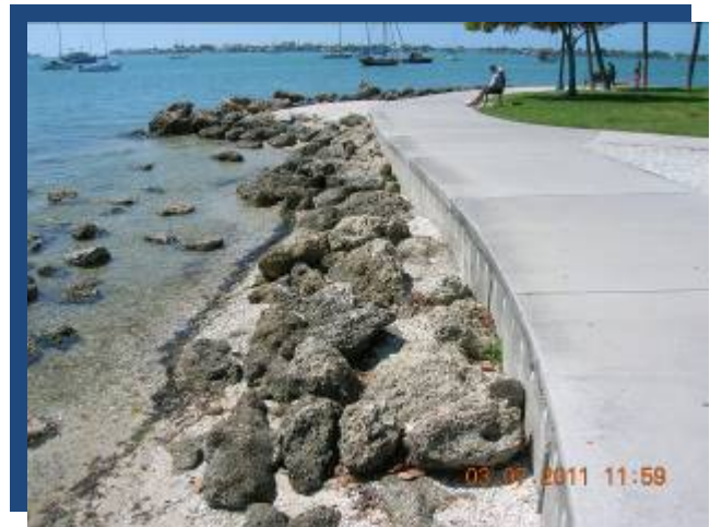
Photograph 12 Rock Armor along East Shoreline
