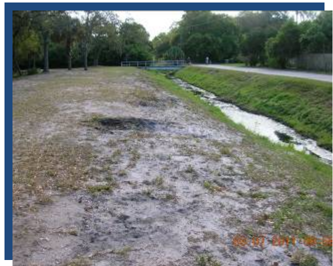
Photograph 29 Ditch Running along Southern Boundary of Park Where Side Slopes Will Be Pulled Back and Planted
