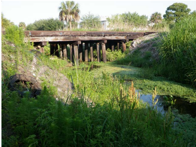
Figure 4-20 SMP2-Erosion along the Waterway on the South Side of Myrtle Street, West of Leonard Reid Avenue
