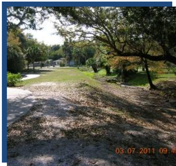
Photograph 28 Facing Southeast along Ditch Coming from Royal Palm Avenue Where Side Slopes Will Be Pulled Back and Planted
