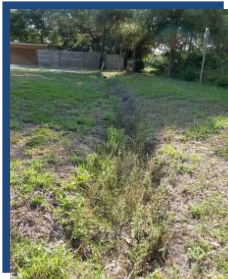
Photograph 31 Ditch Adjacent to Private Properties on the South Side of 47 th Street
