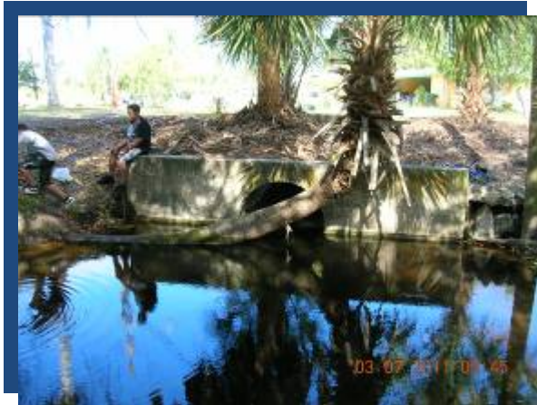
Photograph 23 Culvert and Ditch on West Side of Park Draining Gary Street and Royal Areas to the West Palm Avenue
